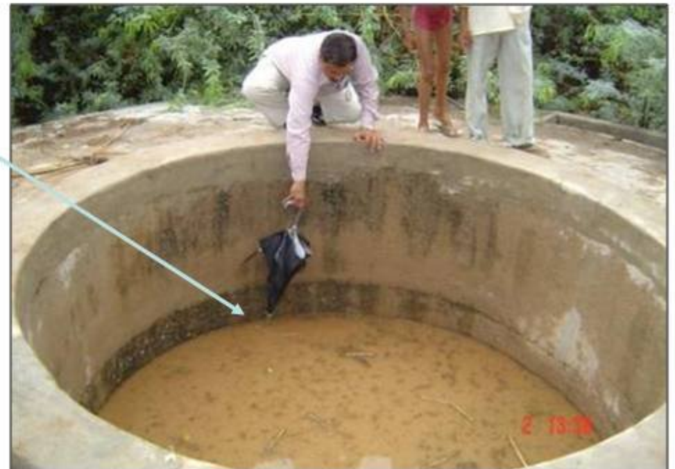
Well recharging structure
